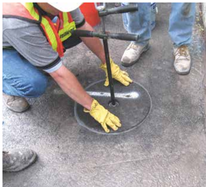
Being able to put the core back into the roadway or sidewalk can save hours of road closure time and thousands of dollars in repaving costs for each repair.
