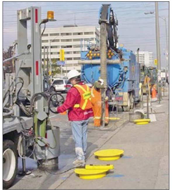
Potholing conflicts in advance of HDD with coring truck in foreground, vacuum truck in background, yellow safety road plates to cover hole between operations and several cores awaiting reinstatement.
