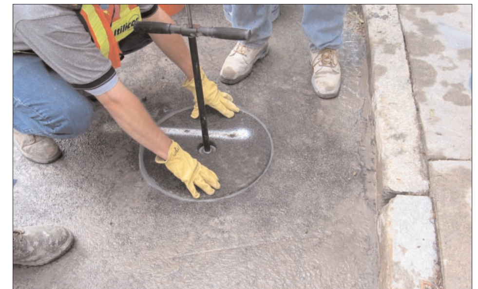
Once the core is reinstated, the road can be re-opened in about 30 minutes.
