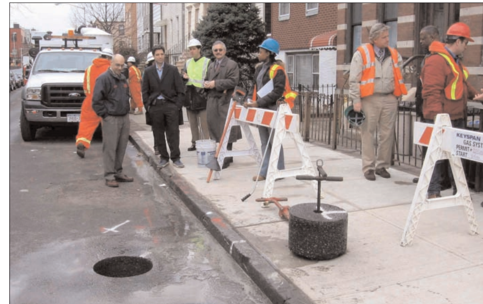
NYC DOT workers with a 13-in. asphalt core on a Keyspan site.
