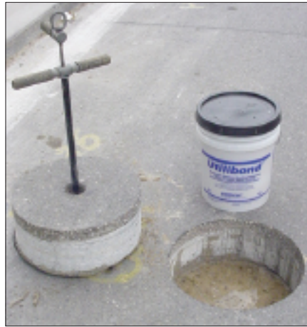
Here, an 18-in. core is removed and set aside for reinstatement later.
