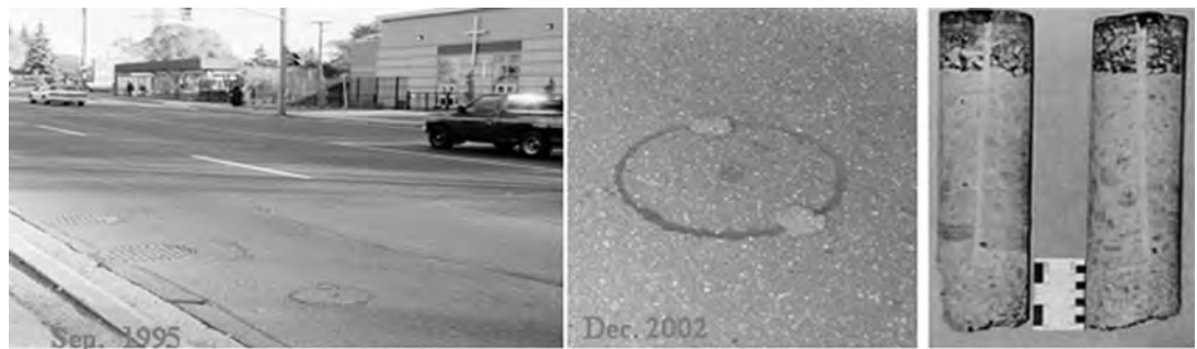
Figure 5: To test the effectiveness of the bond, Golder cut satellite core samples through the kerf of previously reinstated cores. These samples (right) showed perfect and complete bonding or adhesion of the Utilibond to both the surface of the core or coupon and the surface of the remaining pavement, as well as excellent ‘cohesion’ through the joint itself. The light grey line in the photograph is Utilibond, showing excellent bonding of the asphalt–concrete core (central area) to the undisturbed pavement (outer layer) with complete infilling of voids in pea gravel (bottom). The core, which is directly in the wheel path of a transit lane of this arterial road, showed no deflection from the time it was first reinstated in September 1995 (left) to December 2002 (centre) notwithstanding the fact that, during the seven-year interval, more than 145,000 transit buses and 13 million commercial and other vehicles have passed directly over the keyhole with no apparent weakening or other degradation of the reinstated core or the adjacent road system or paved surface
