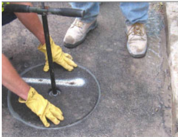
After the bonding material has been poured into the hole, the core is reinstated and carefully adjusted to be level with the rest of the pavement
