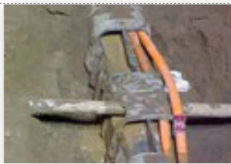
HDD drill rod penetrates fibre-optic cable.
