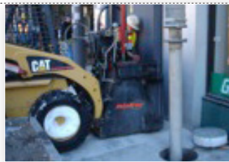
Minicor skid-steer coring attachment cores inspection hole through pavement to allow vacuum excavation.
