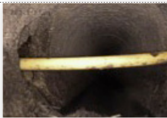
2-inch HDPE gas distribution line (yellow) cross-bored through sewer lateral.
