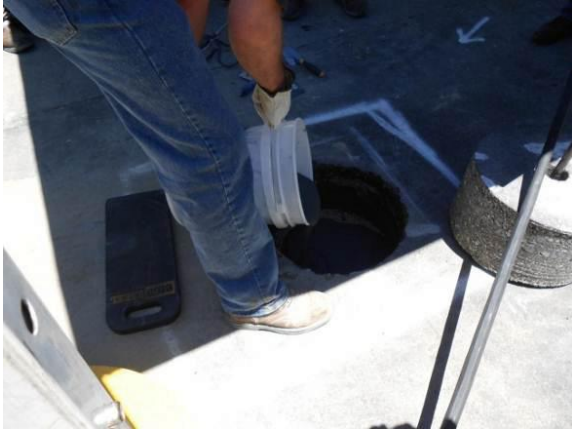
A grout-like bonding agent (Utilibond) was poured into the hole. The extracted core, shown on the right side of this photo, is ready for placement.
