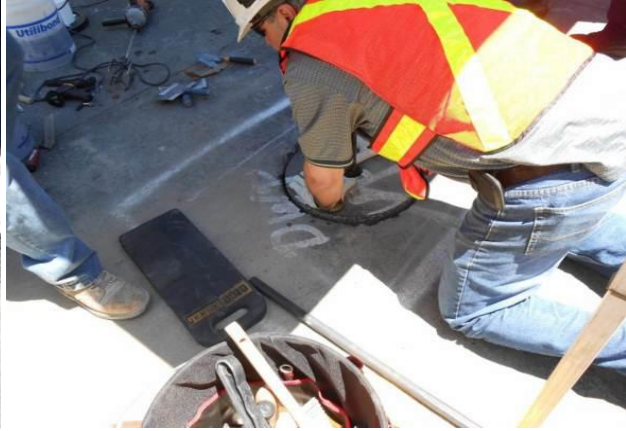
The core is placed into the hole, then wiggled back and forth, forcing the bonding agent up the sides and center of the donut-shaped core. Marks spray-painted before coring assured proper alignment of the core with the rest of the pavement.
