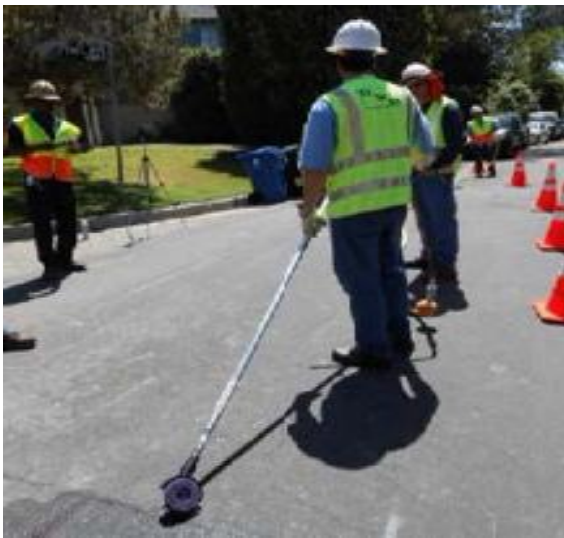
A long-handled, air-powered grinder with plastic abrasion disk was used to prepare the pipe surface for wire bonding.
