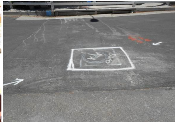
The restored hole was ready for traffic in less than one hour. (In lower temperatures more time is required.) This picture was taken the next day.
