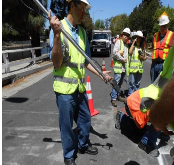
Another long-handled tool was used for exothermically welding the anode to the pipe. (In this case, the attachment was to a steel pipe. A brazing method is needed for attachment to a cast-iron main.)
