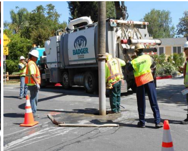
Vacuum excavaton was then performed using a high-volume unit equipped and water jets lances.
