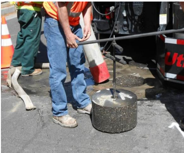
The core was lifted from the hole by two persons, using a special tool that grips the center pilot hole.
