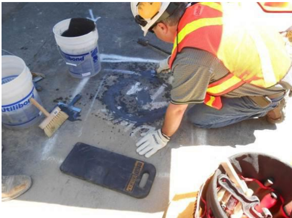
Standard cement mason tools and techniques were used to finish the surface.
