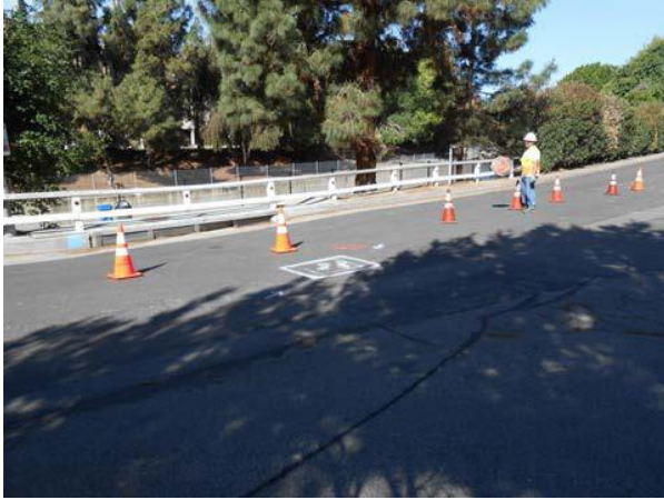
Traffic control by LADWP. The hole location was pre-marked and cleared for excavation.
