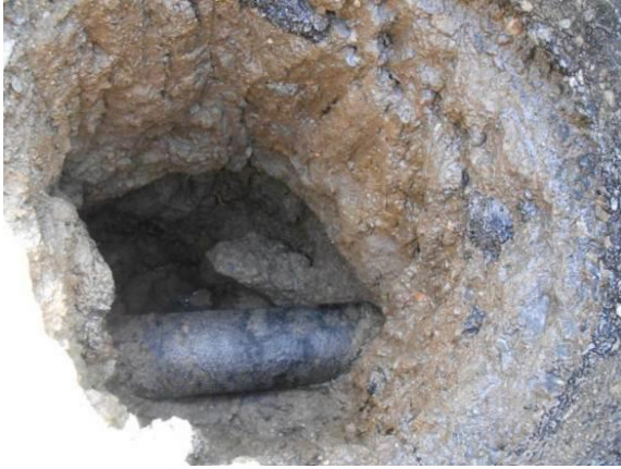
This shows the completed excavation. The hole extended several feet below the main to allow proper burial depth for the anode.
