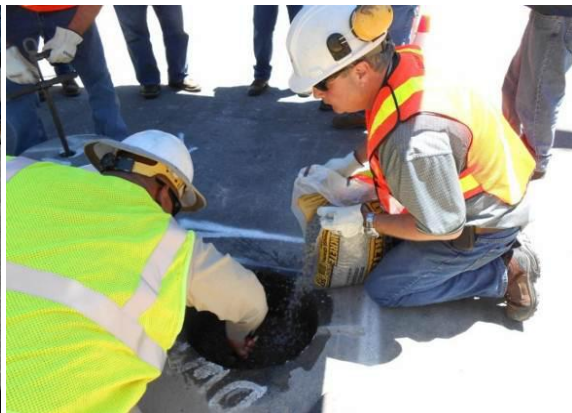
After backfilling using conventional methods, a layer of pea gravel was placed for leveling. This was followed by a dry-fit test to verify that the excavated core would be level with the adjacent pavement.
