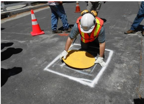
The excavations can be plated without a backhoe or other equipment. The plate has an underside ring that extends into the hole, preventing it from sliding. Plates are available that lock in place.
