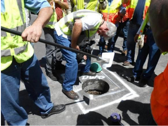
A corrosion protection patch was placed over the weld using another long
